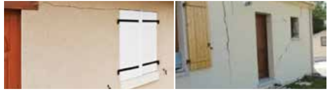
Figure 8: cracks as a manifestation of disorders due to swelling-shrinkage phenomenon
